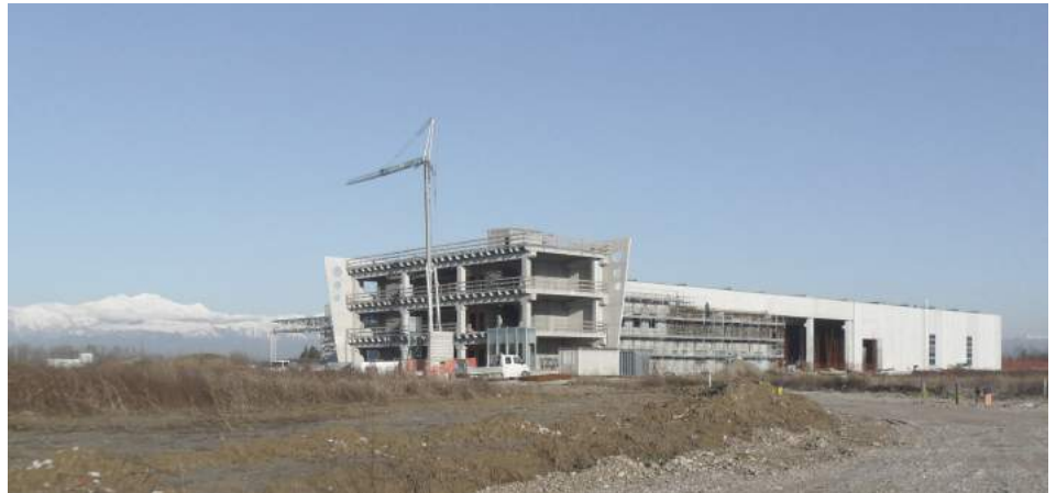
The building site of the pumps/decompressors facility in the Fiumesino industrial estate
